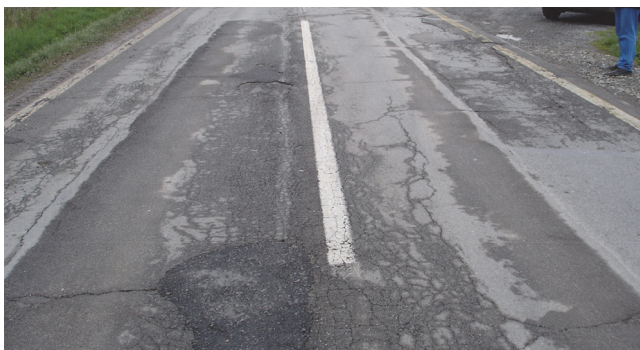
Figure 1. Asphalt surface deteriorated by use
