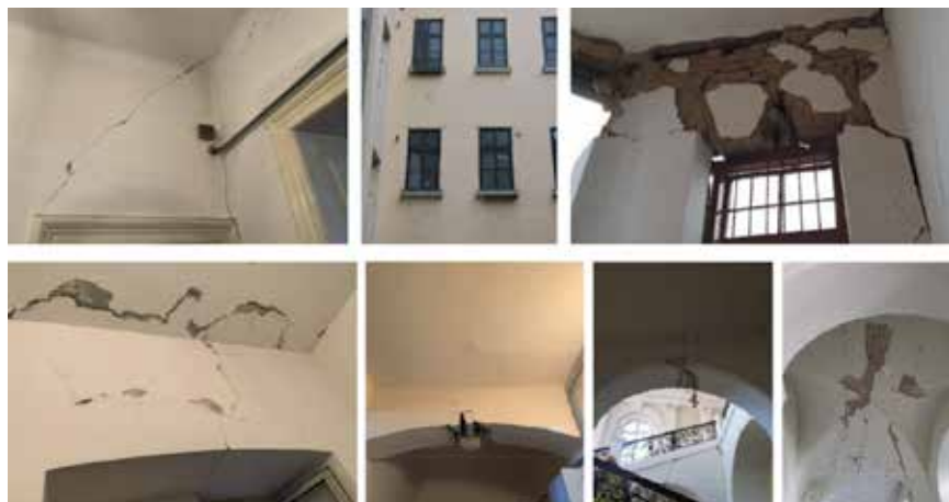
Figure 23. Lintel damage: diagonal and vertical cracks [39]
