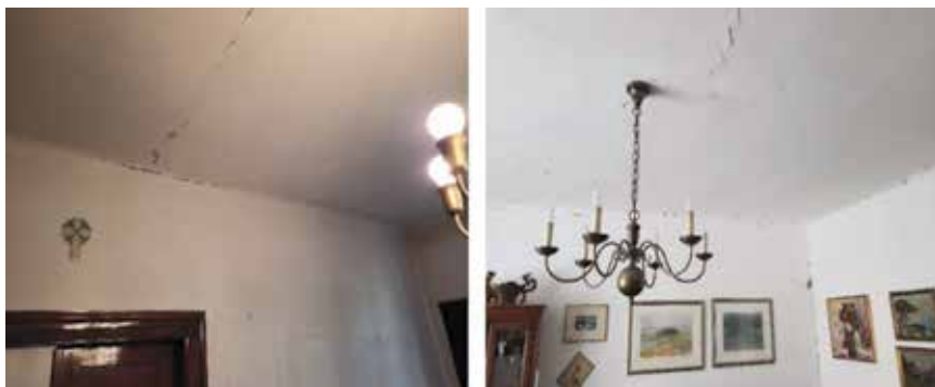
Figure 24. Cracks at ceilings [39]
