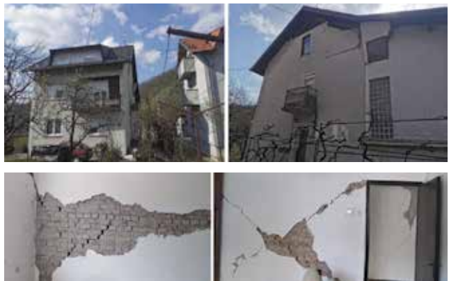
Figure 29. Damage to houses at LB Dankovec, CD Gornja Dubrava (photo courtesy of Luka Božić and [39])
