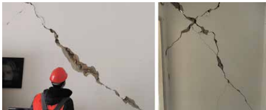
Figure 1. Masonry damage caused by Zagreb earthquake of 22 March 2020
