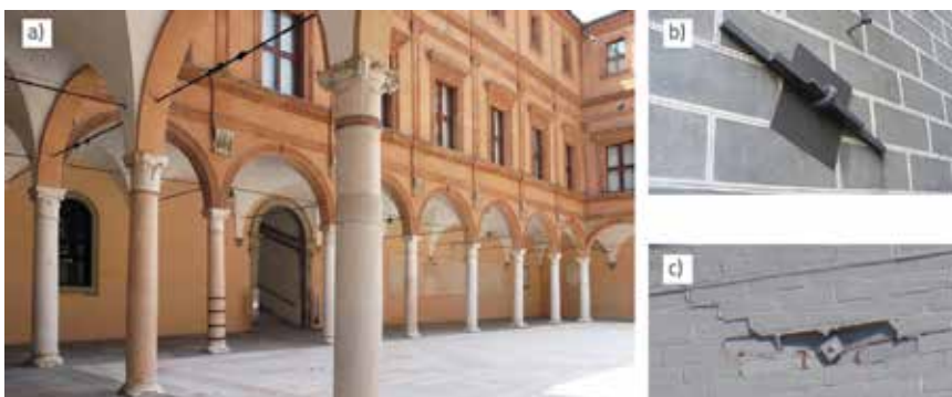
Figure 9. Steel tie rods: a) Example of old and recent tie rods (above old ones); b) Tie rod anchorage detail; c) Typical mode of failure
