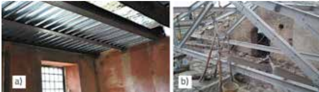
Figure 4. Lightening of structural system: a) replacement of a heavy wooden floor structure with composite structure; b) replacement of wooden roof truss with steel truss
