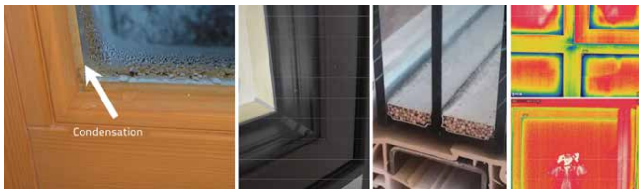
Figure 16. Condensation of water vapour at the glass edge (left), composite and aluminium glass edges (centre), thermogram of thermal bridge at glass edge (right)
