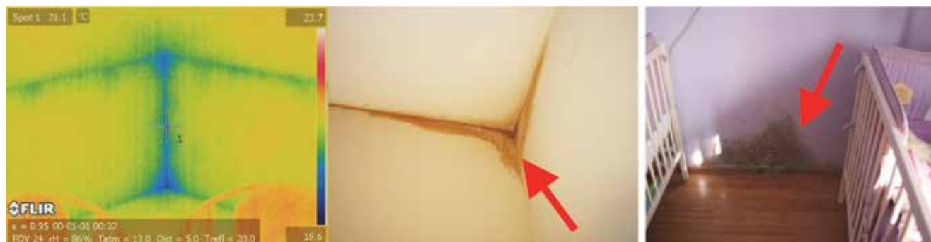
Figure 13. Thermogram of thermal bridge in the existing NZEB family house in Zagreb (left), consequences of thermal bridges (centre and right)
