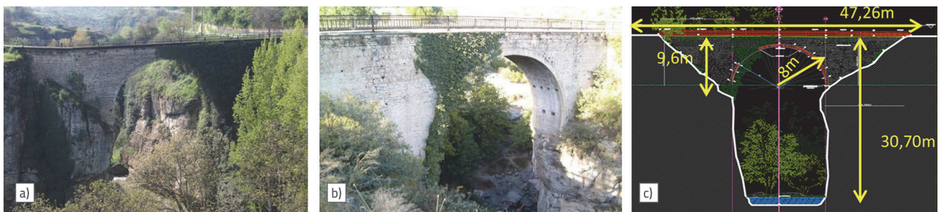
Figure 1. View Of The Historic Tokatlı Bridge (a) Upstream, (b) Downstream View, (c) Building Survey [41]
