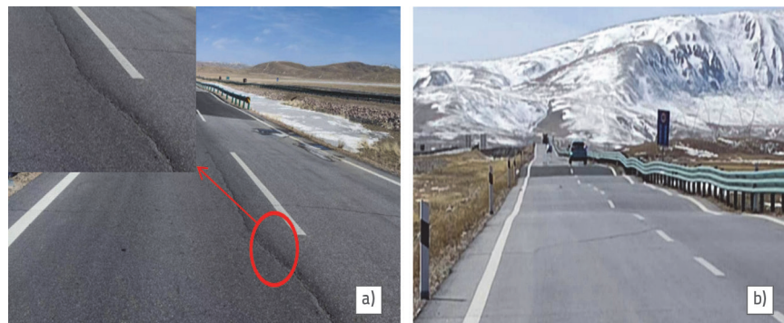
Figure 2. GongYu expressway road condition: a) Longitudinal crack; b) Uneven road settlement
