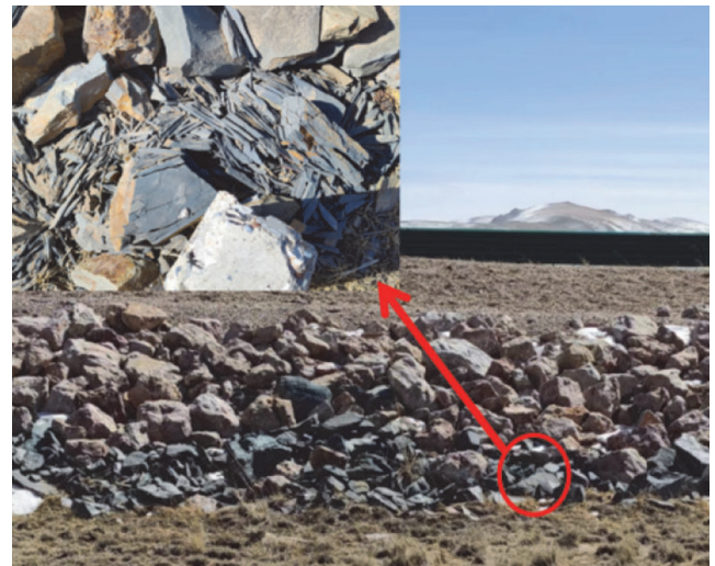
Figure 3. Rock weathering on the slope of Gongyu expressway
